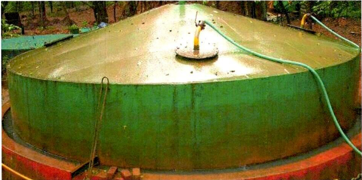
Biogas Plant at college
