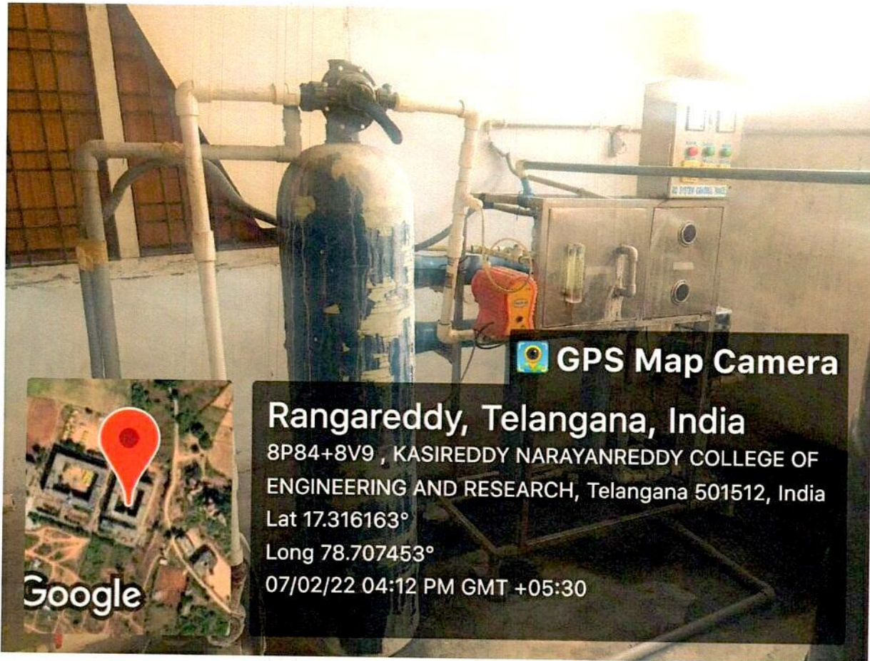
RO water plant.
