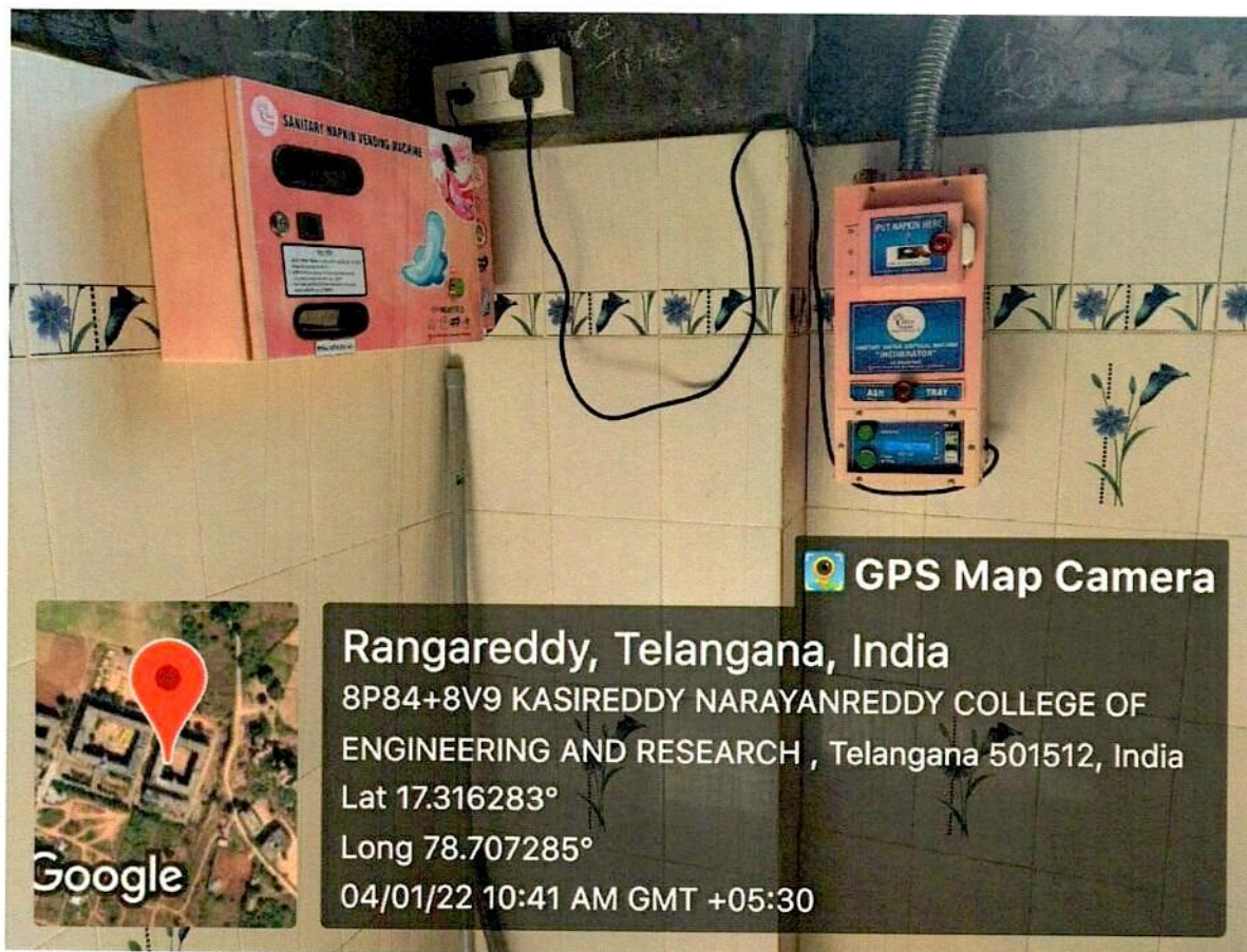
Vending and burning machine in the institution premises
