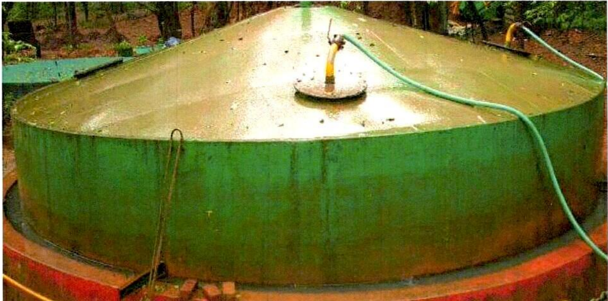
Biogas Plant at college
